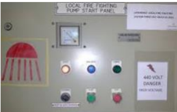
Figure 2 Local firefighting pumps panel [3]
